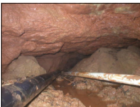
The water disposal system
